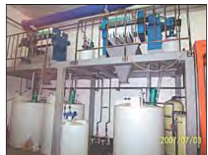
Waste water treatment plant.
