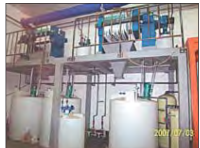
Waste water treatment plant.
